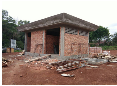
TNB Sub Station
