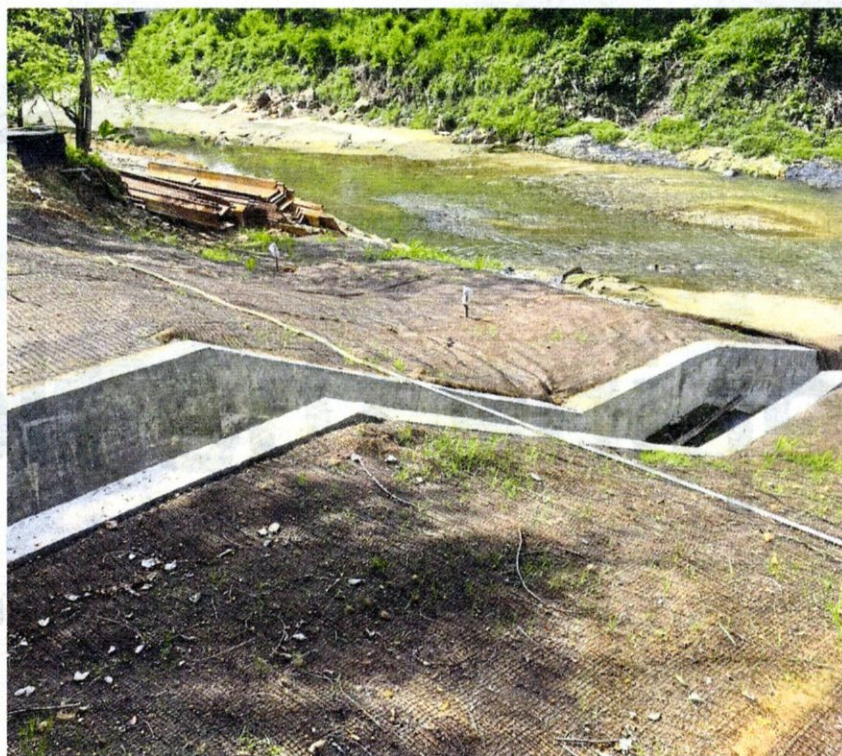
So far, the most pressing problem of the collapsed bank and monsoon drain at Jalan PJU1A/26D has been repaired.
