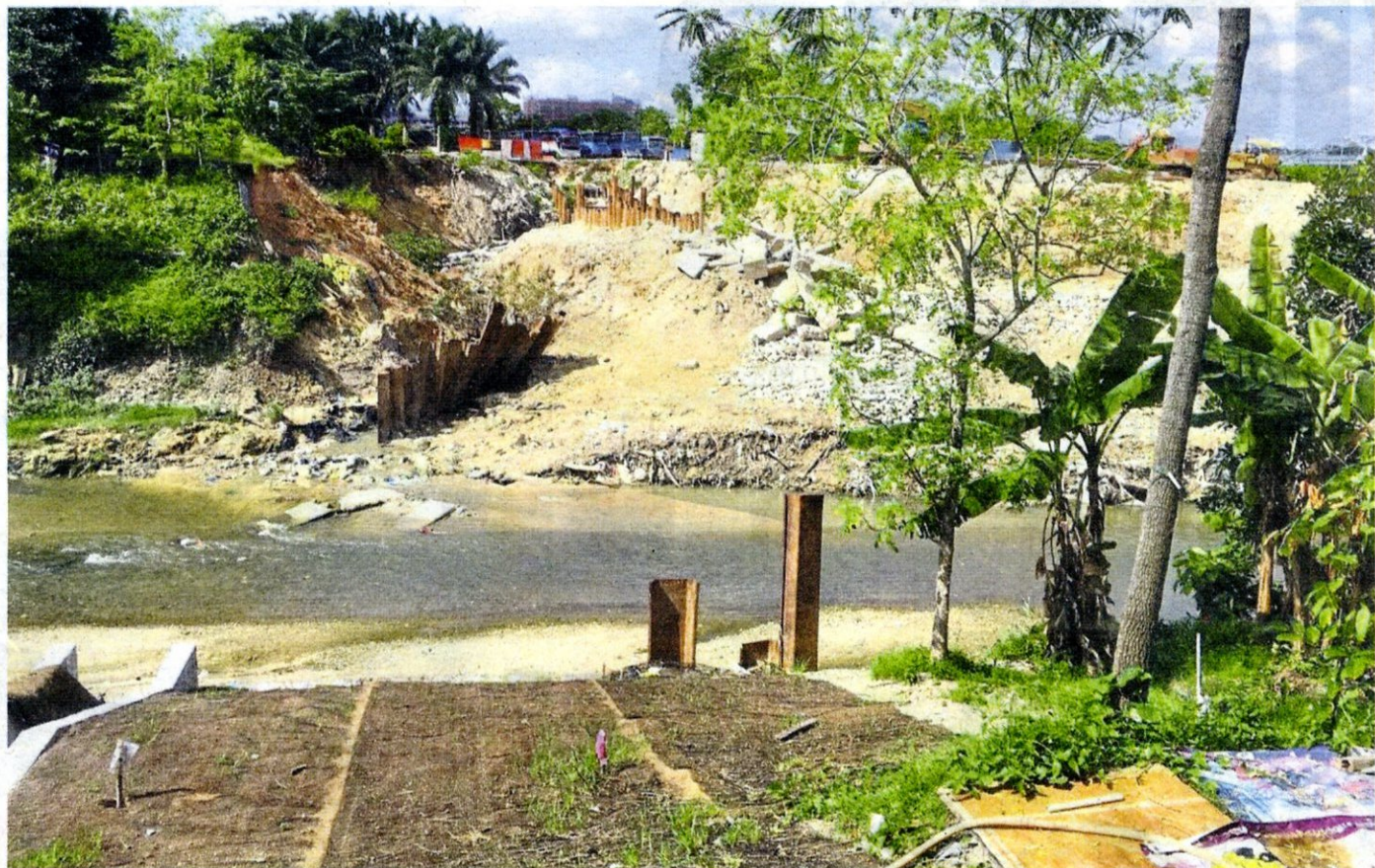
Opposite Jalan PJU1A/26D, sheet-piling work has been partially done, according to local resident Foo Teck Leong.
