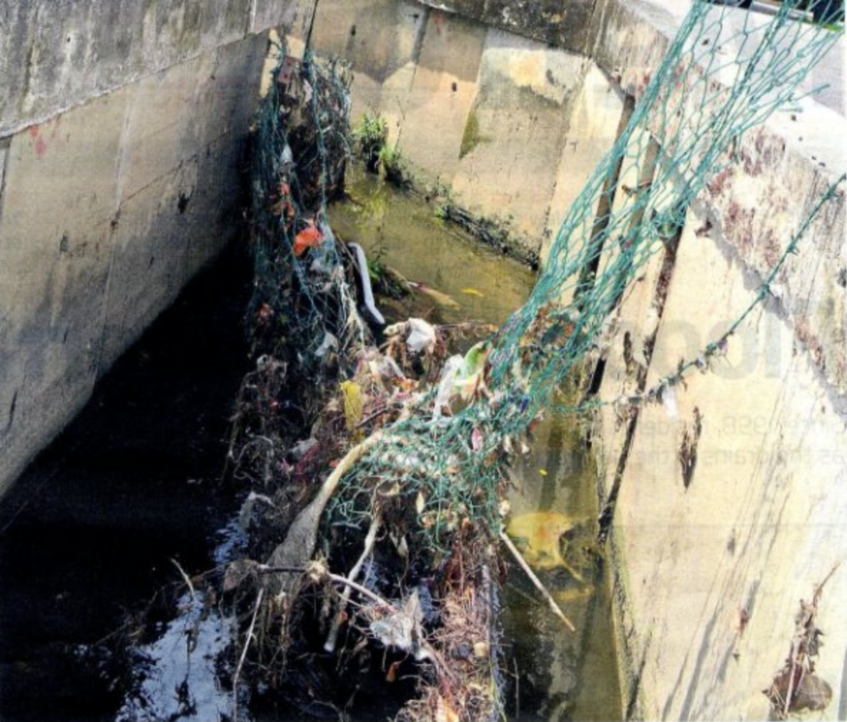
Poor maintenance of the monsoon drain in Jalan Batu Unjur 6 in Taman Bayu Perdana with a collapsed fence is trapping rubbish and impeding water flow.
