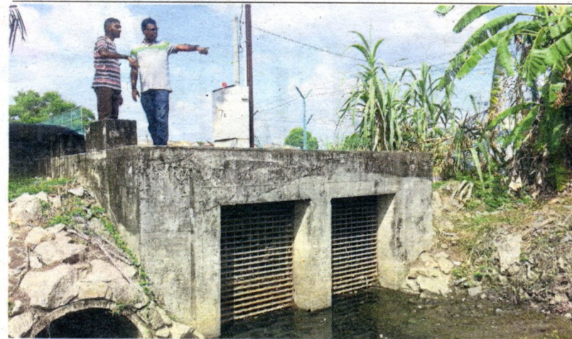
Desmond (right) and Rubenraj checking the condition of the pump house at Taman Sungai Jati in Klang.
