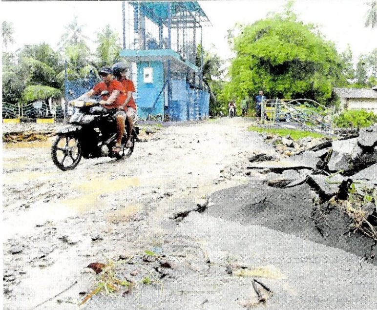
The damaged road in Kampung Raga, Yan, yesterday.
