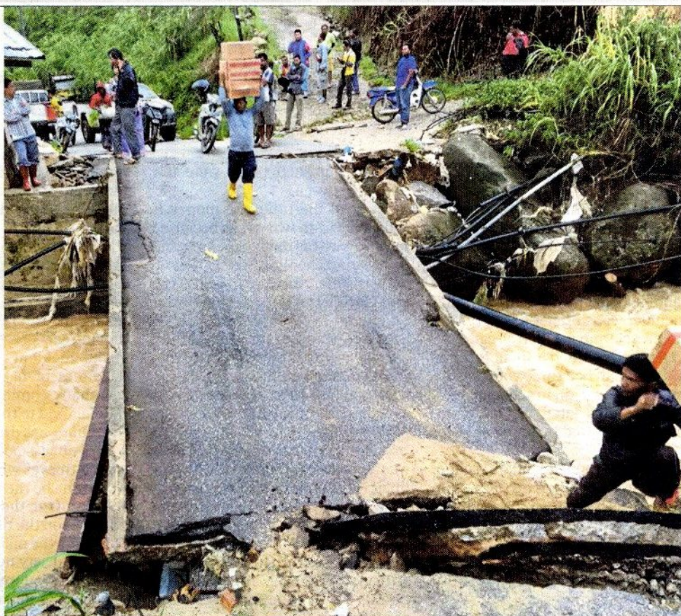
Villagers making their way across the collapsed bridge over Sungai Ulu Telom in Cameron Highlands yesterday. Pic courtesy of Fire and Rescue Department
