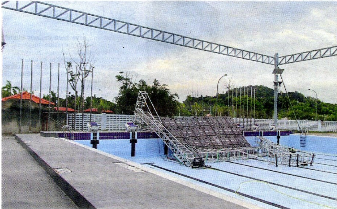
For the record: The electronic scoreboard of the National Sports Council's swimming pool at the Tuanku Syed Putra Stadium was damaged during the thunderstorm in Kangar. - Bernama
