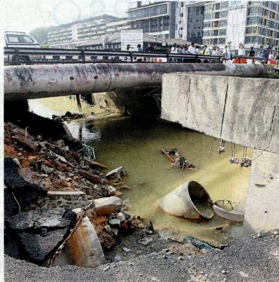
The Jalan Bukit bridge in Kajang will be elevated to ease water flow along Sungai Jelok while reinforcement work will be done to repair the sidewalks that had recently collapsed because of erosion. — AZHAR MAHFOF/The Star
