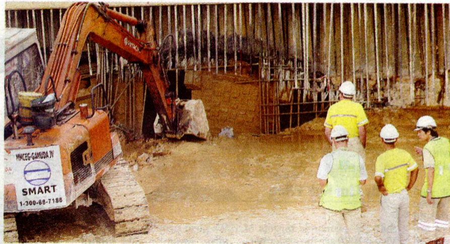
An excavator clearing the way to let workers out of the boring machine at Taman Desa.
