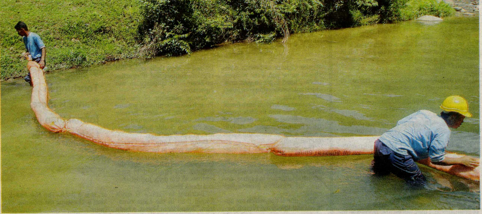
Two Syabas workers placing booms to prevent the spill from spreading further.
