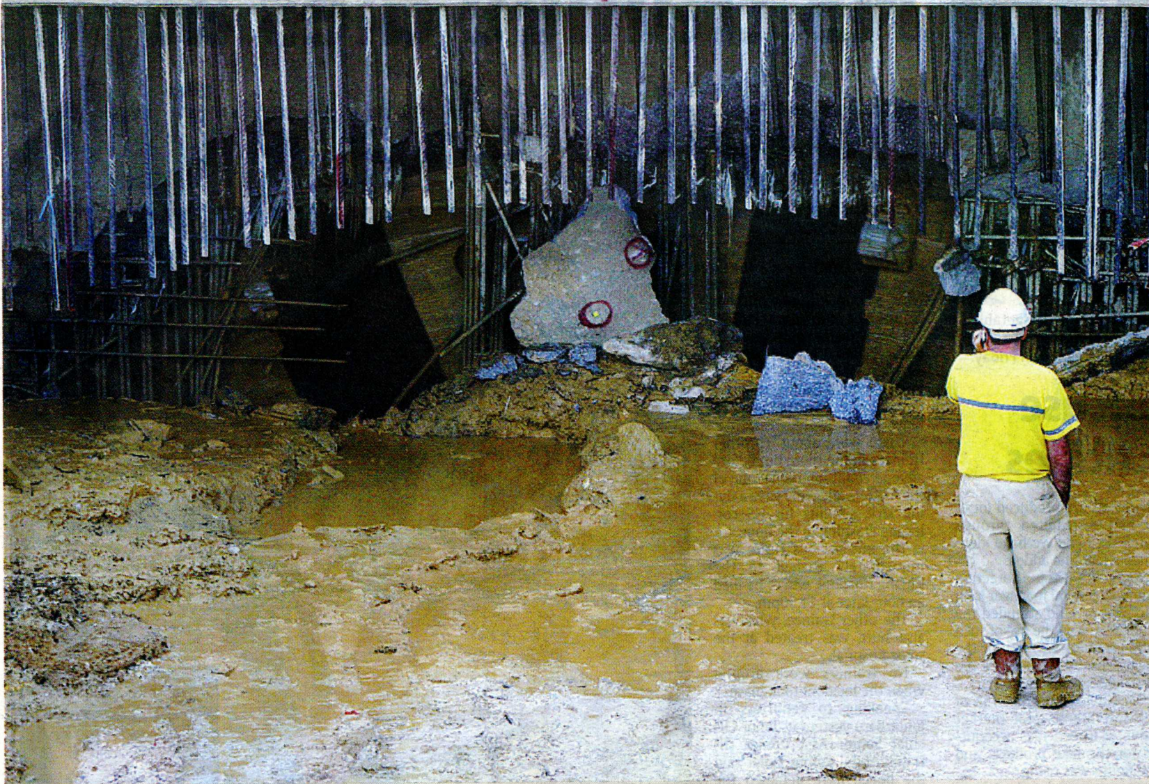
A WELCOME SIGHT: A worker looking at 'Gemilang' after it emerged from the ground at Taman Desa yesterday.
