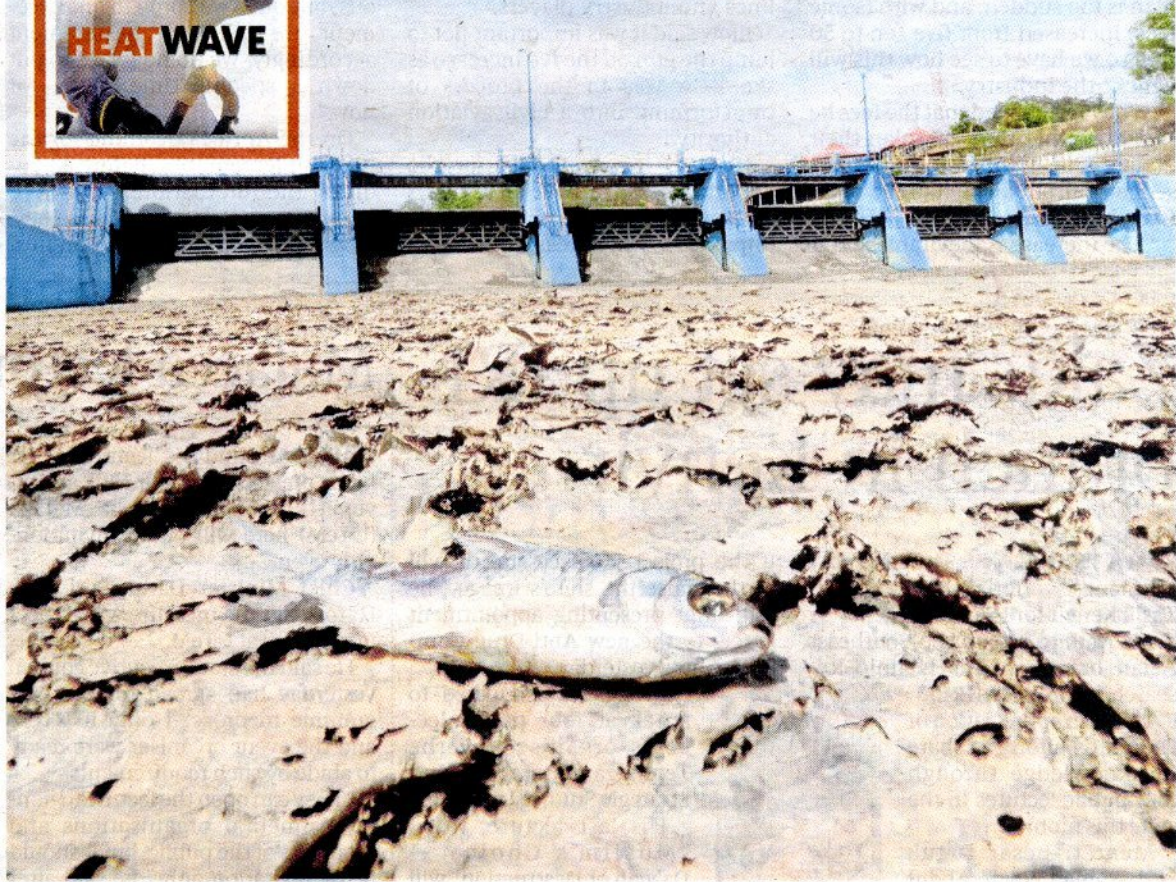
Mudcracks in front of the Timah Tasoh Dam gate in Kangar on Tuesday. Pic by Eizairi Shamsudin
