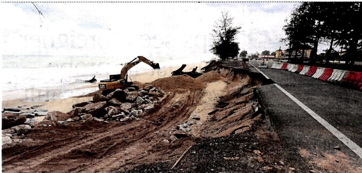
The Pantai Teluk Lipat main road is closed to vehicles while roadworks to control erosion is ongoing. Pic by Rozainah Zakaria
