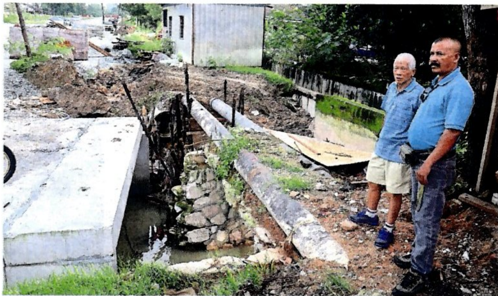
The construction of Jalan Harapan's 'missing link' to the Sprint Highway contributed to the flash floods as heavy rains have washed the construction debris into local drain systems, clogging them up.
