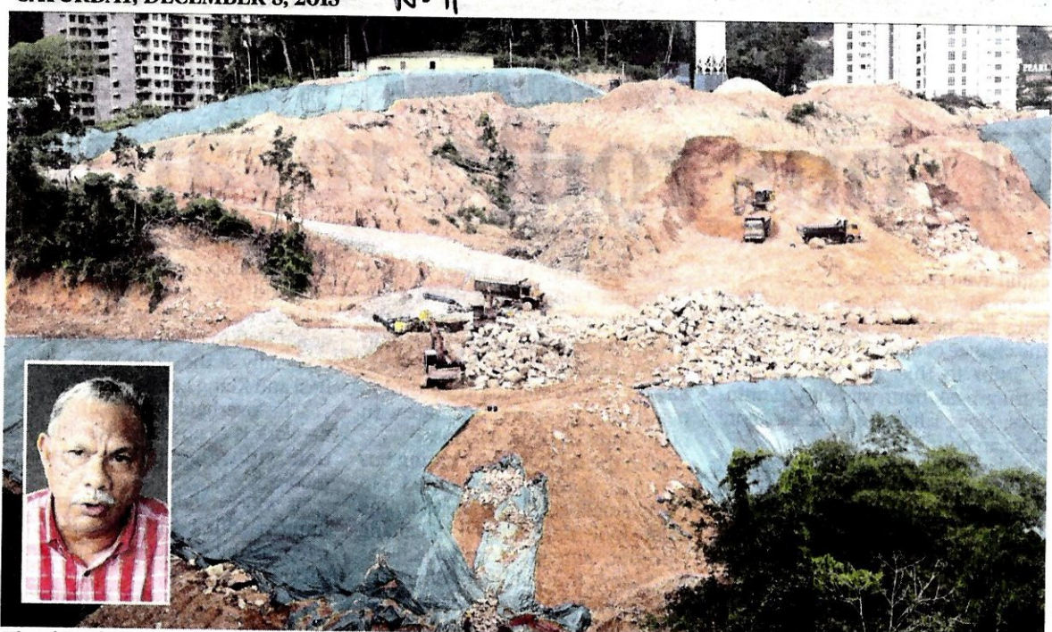
The site of the development project that caused a flash flood in George Town. Pic by Zulaikha Zainuzman (Inset) Bayan Lepas assemblyman Nordin Ahmad has expressed his dissatisfaction with the state government.
