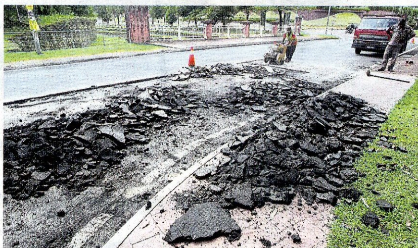
The crumbled stretch of the road near Jelutong Plaza at Bukit Jelutong has been dug up for repair works.
