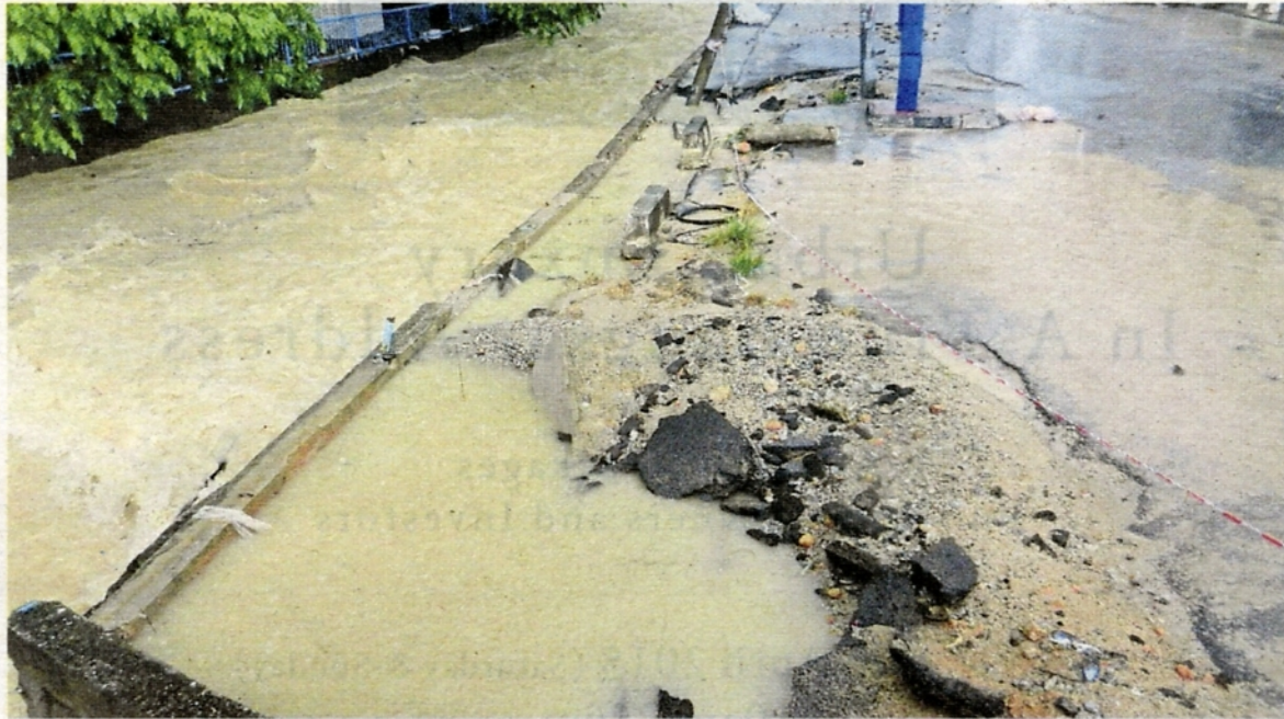
Cause of floods: The embankment is badly damaged, but has yet to be fixed.
