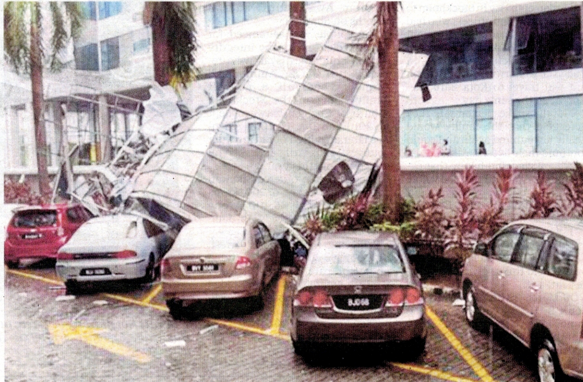
A building at the Bukit Jelutong Industrial Park is damaged by the heavy storm that struck Shah Alam and Kajang yesterday, leaving a trail of toppled trees and power outages. Pic courtesy of Fire and Rescue Department
