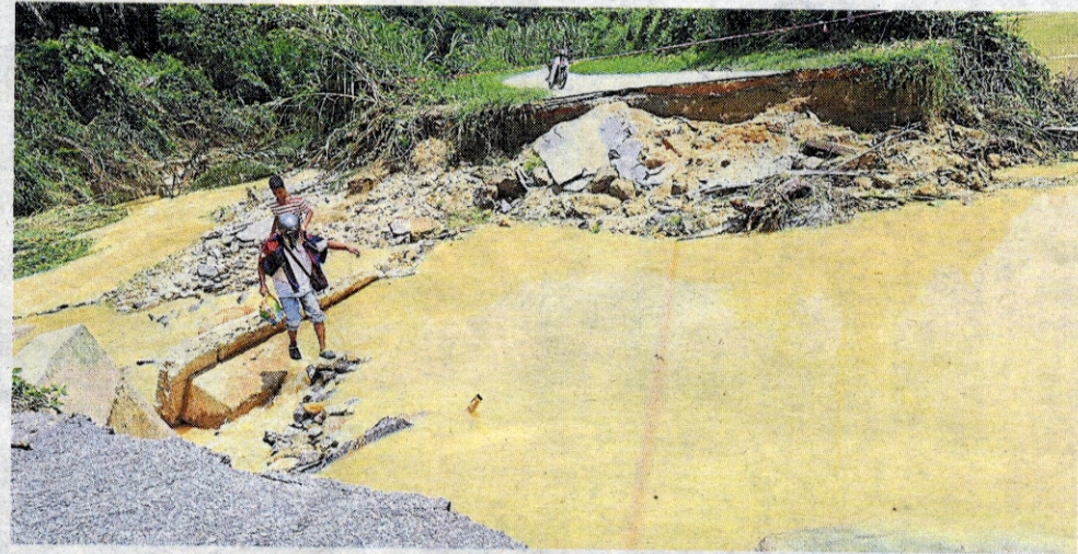
Fallen crossing: The Sungai Cincin bridge that linked Chenderiang town with Kem PLKN Sentosa was swept away by flood waters.
