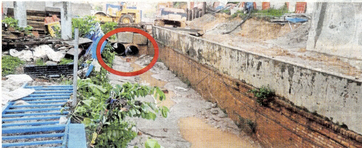
A temporary culvert (circled) at the main drain in Jalan Semantan is believed to have blocked the flow of rainwater.
