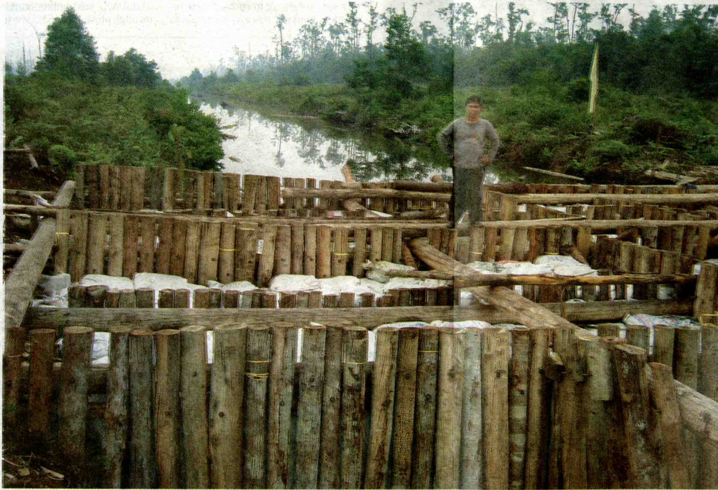
Sandbags fill the spaces between rows of logs that make up a block in a Central Kalimantan canal — Picture by Faizal Parish, GEC.
