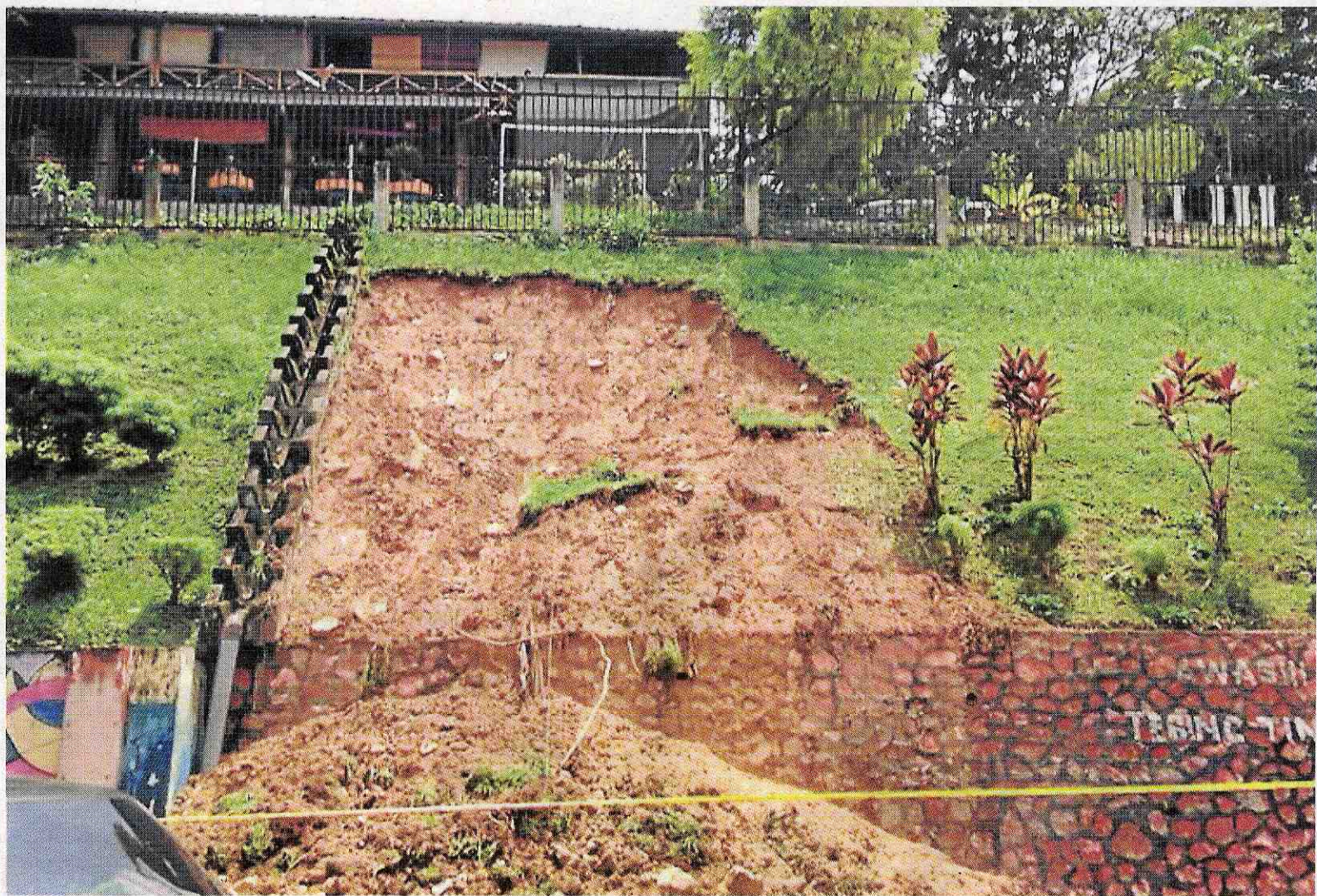
Dangerous situation: The damage caused by the landslide at SMK Bangsar following the downpour on Thursday evening.
