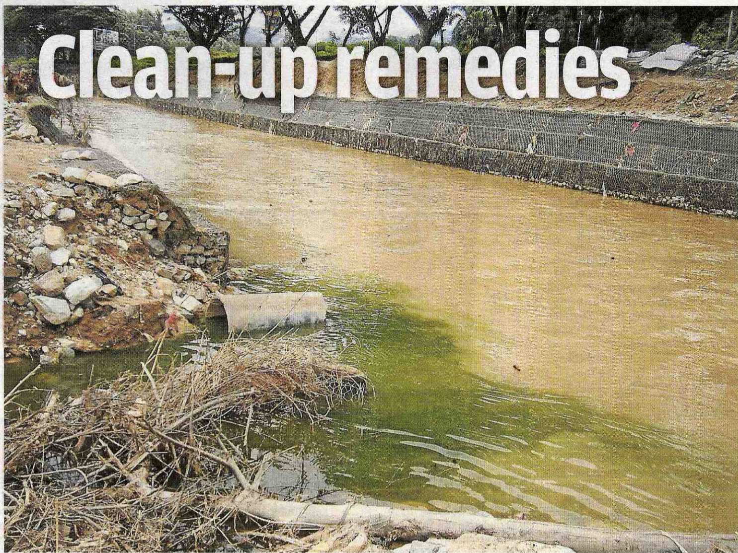
Hidden danger: Sillage, coloured green by algae which proliferate due to the presence of sewage, flowing directly into Sungai Klang from the Keramat neighbourhood in Hulu Klang, Kuala Lumpur. This source of pollution is often overlooked in river-cleaning efforts. – Filepics
