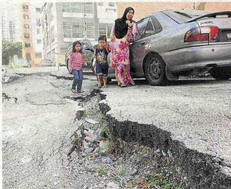
Accident waiting to happen: Damansara Bistari resident Ramlah Saad and her grandchildren have to be careful each time they walk along the collapsed road.
