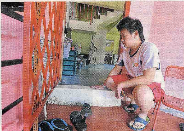
No reprieve: A one-foot retaining wall was not enough to prevent water from entering the house of Ryan Fong Rui Chuan (above).
