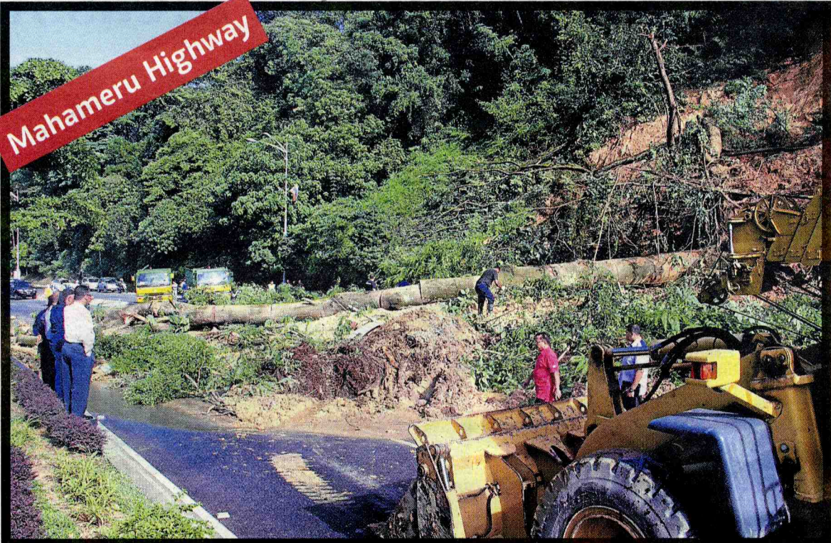
Bulldozers are deployed to clear the debris after the landslide near Mahameru road towards the Jalan Pahang roundabout.
