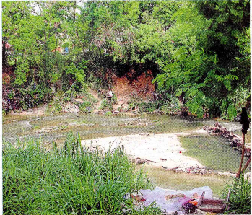
Washed away: Sungai Kayu Ara's riverbank is heavily eroded and needs to be rectified urgently.
