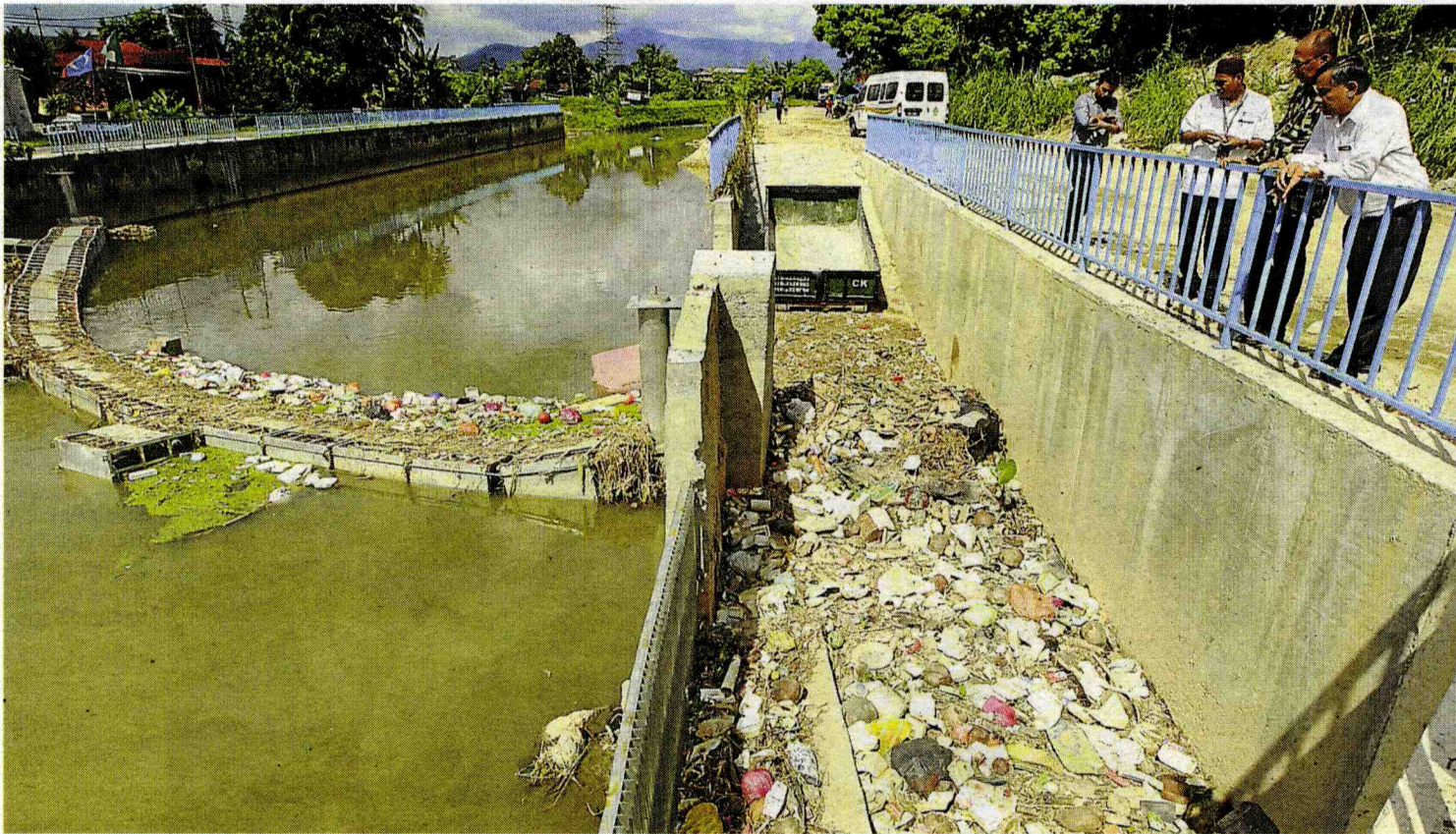
Eyesore: A floating boom in Sungai Gombak near Kampung Padang Balang in Gombak. Litter is being raked to a section specially built to contain rubbish.
