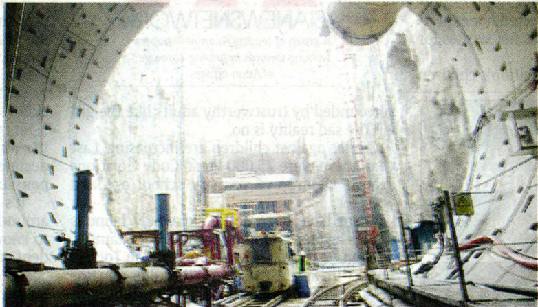
BREAKTHROUGH: North Drive tunnel exit at the North Junction Box where the shared road and water portion meets the stormwater only portion.
