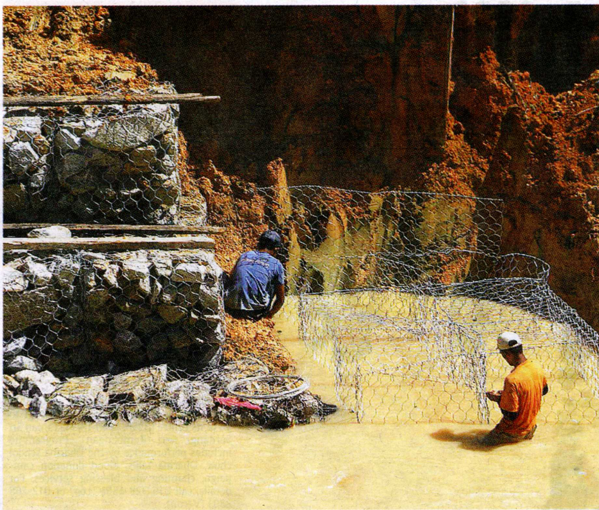
Selangor DID workers working on the gabion wall to prevent further damage of the road.
