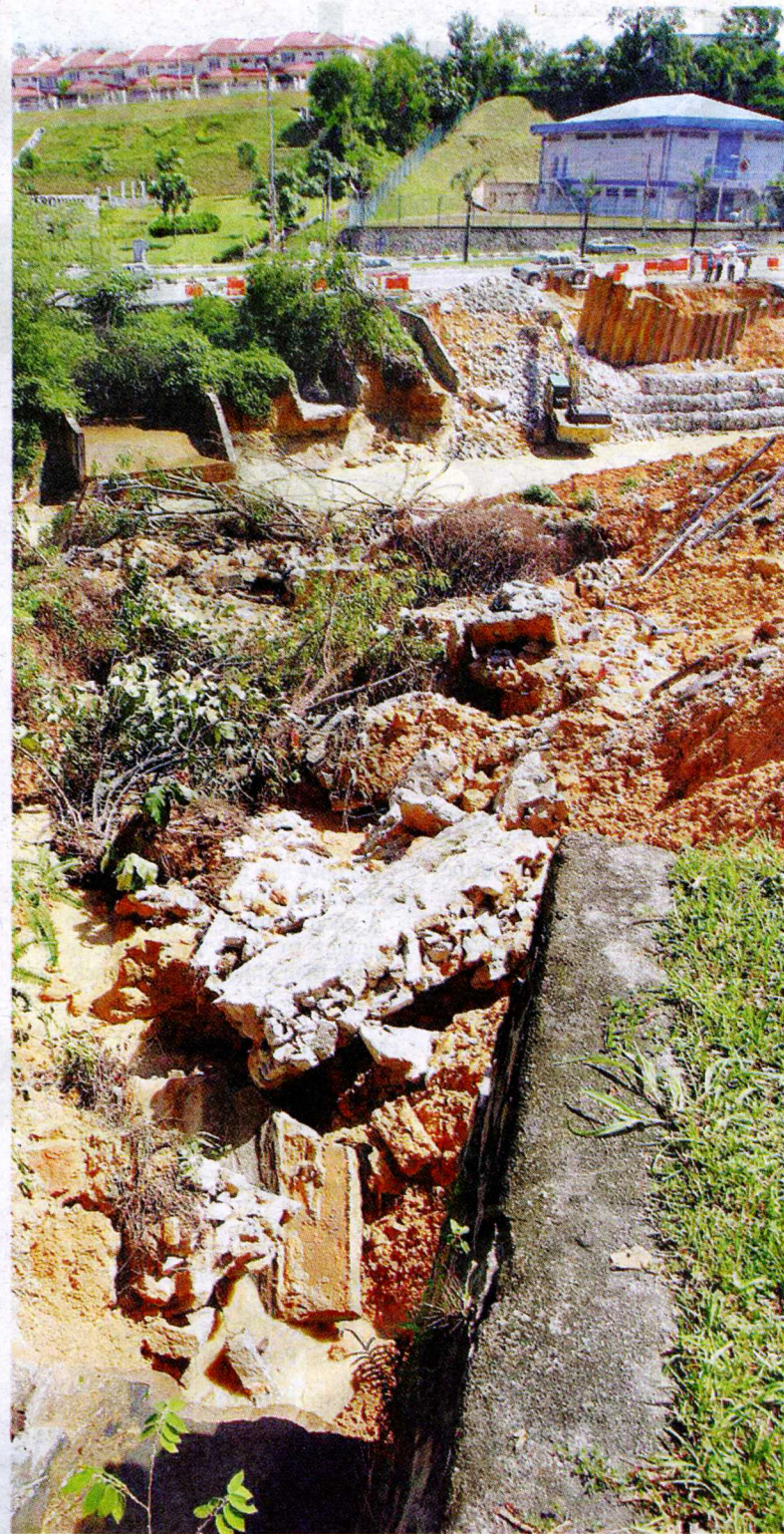
The condition of the road in Bandar Sungai Long, Cheras, after Tuesday's downpour.
