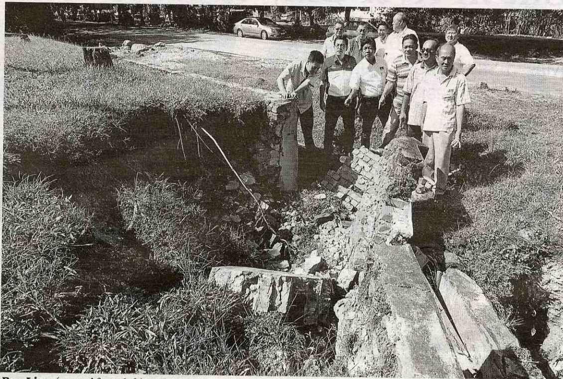
Ben Liew (second from left) and residents of Taman Muda showing the collapsed wall of the drain and soil erosion at the Jalan Bunga Raya Esso petrol station. Pic by Yong Chee Choong
