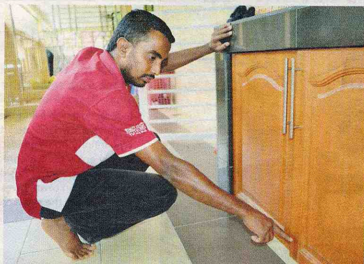
Waterlogged: Thiagarajah pointing out the water damage on his cabinets. — Starpic by Jarod Lim
