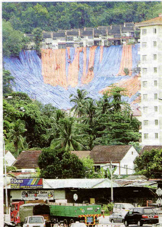
PRECARIOUS: This shot shows the back portion of the houses in Taman Zooview. The authorities covered the site with plastic sheets to prevent further soil movement and said that they are still waiting for the preliminary report
