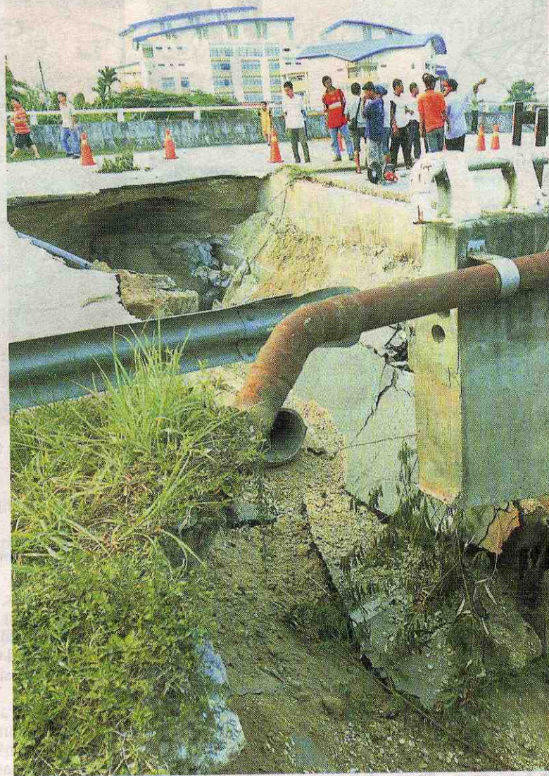
Dangerous drop: The gaping hole is about 12-feet wide, 36-feet long and 10-feet deep. The road is closed to prevent danger to road users.
