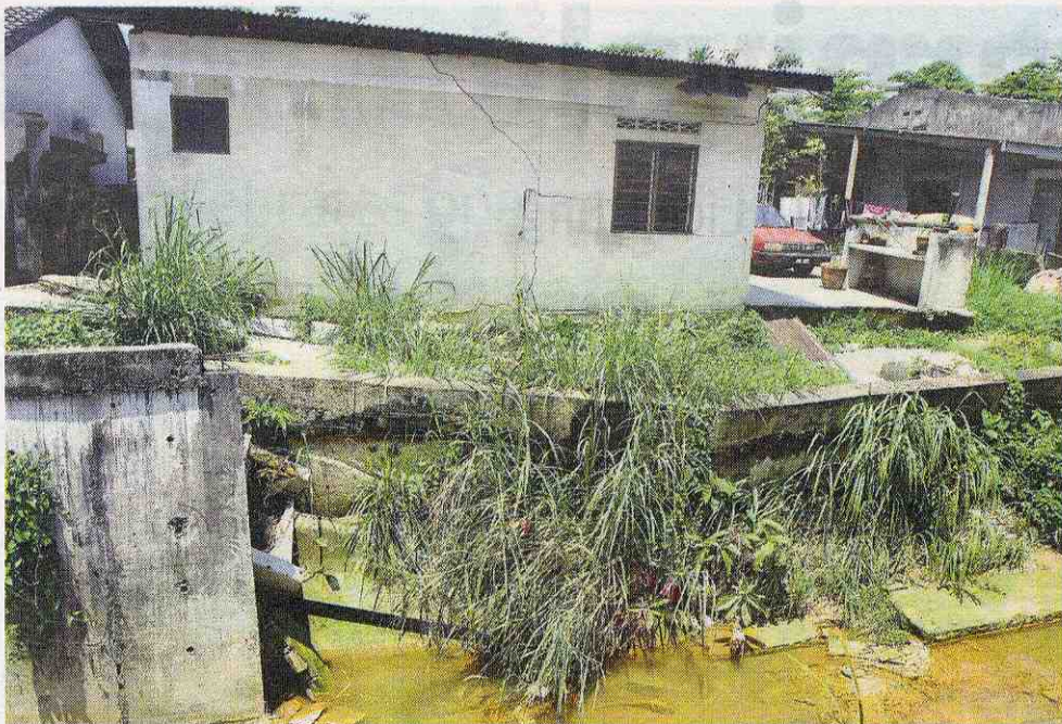
Dangerous: Part of a house in Kampung Desa Aman in Sungai Buloh situated next to the monsoon drain is sinking.
