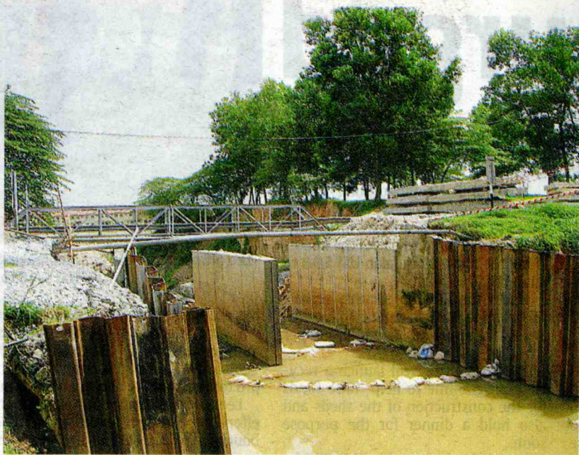
Work is under way to rebuild the bridge in Jalan Reko from a two-lane to a four-lane structure.
