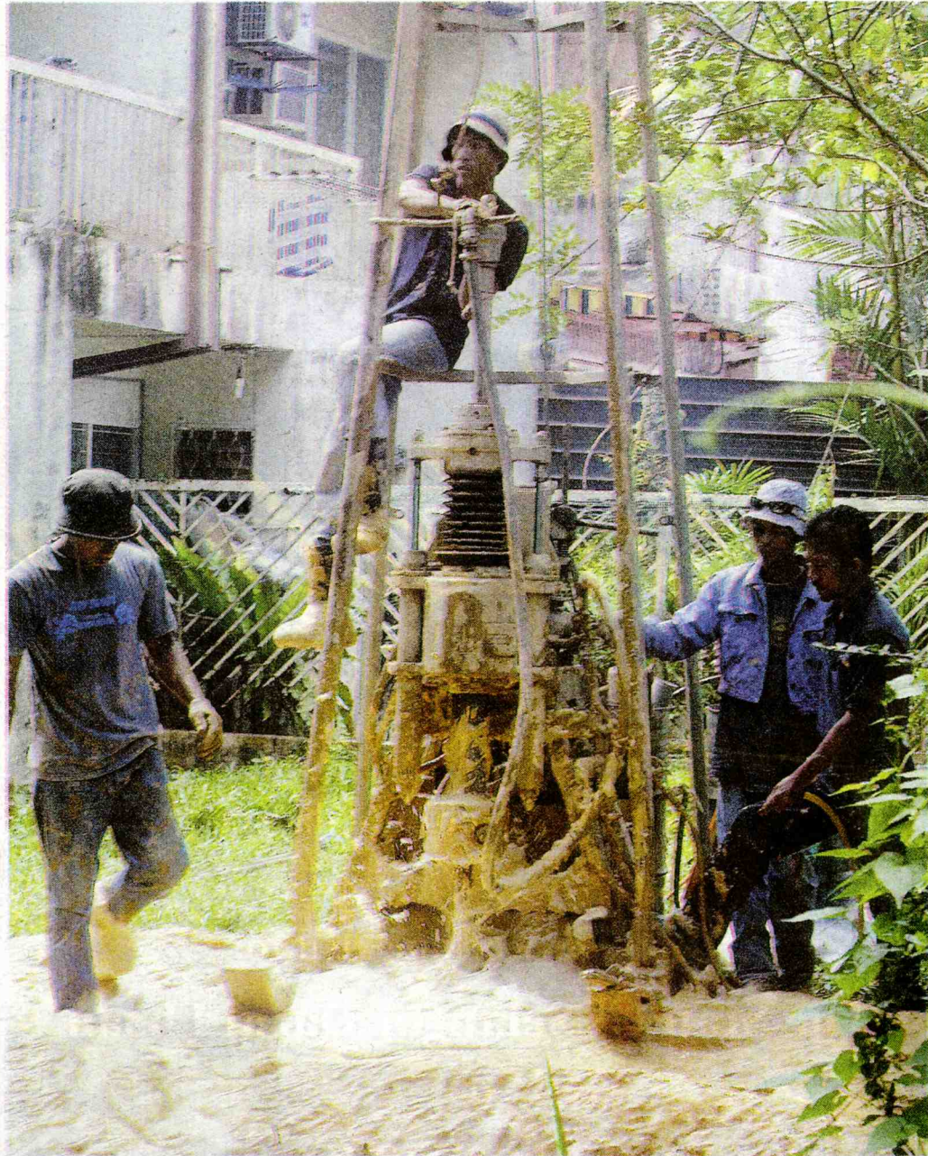
Institut Kerja Raya Malaysia (Ikram) personnel conducting soil evaluation work at a house in Taman Zooview, Hulu Klang, yesterday. — NST picture by Abd Rahim Rahmat
