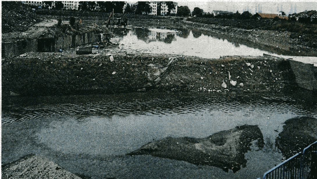
Construction work at this retention pond near Sungai Keroh led to a wall of soil that prevented excess water from the river from flowing into the pond. This caused homes to be flooded. Pic by Nurul Syazana Rose Razman
