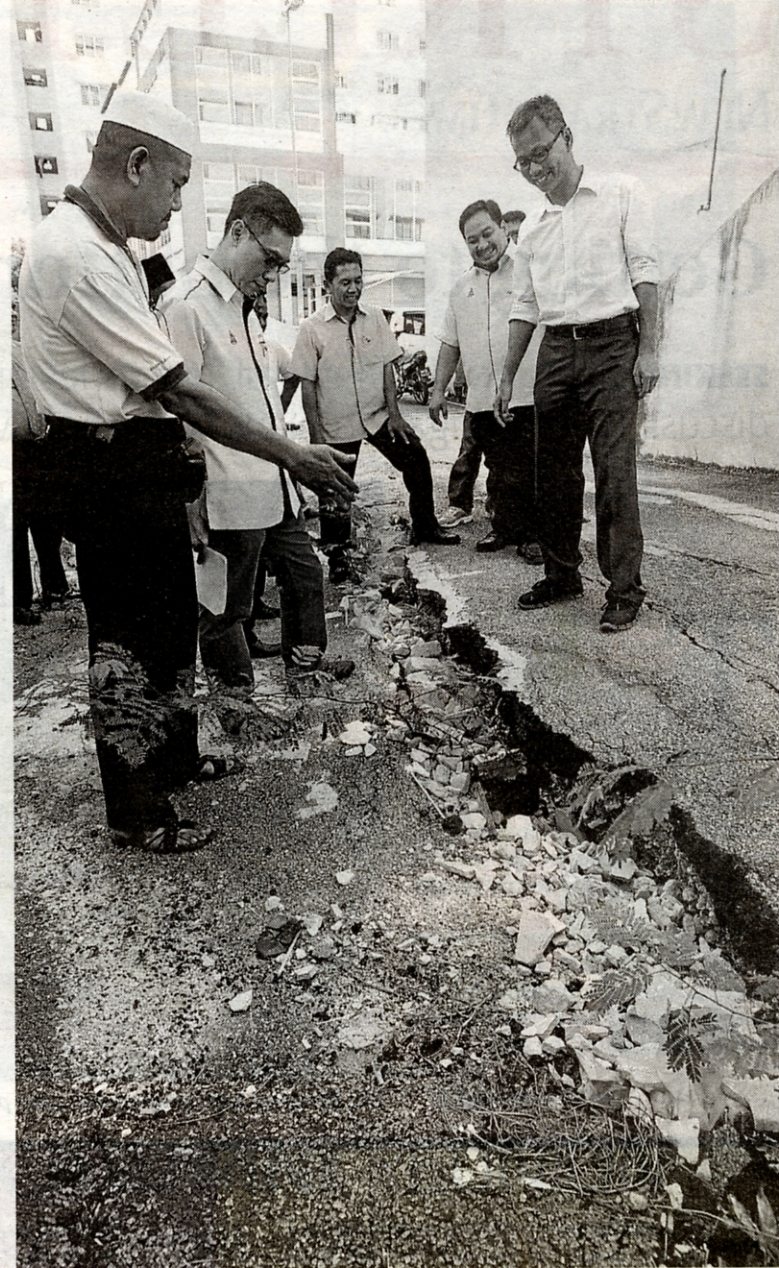
Lee Suet Sen (second from left) checking on the collapsed road at the Damansara Bistari apartment in SS2. Pic by Nashairi Mohd Nawi
