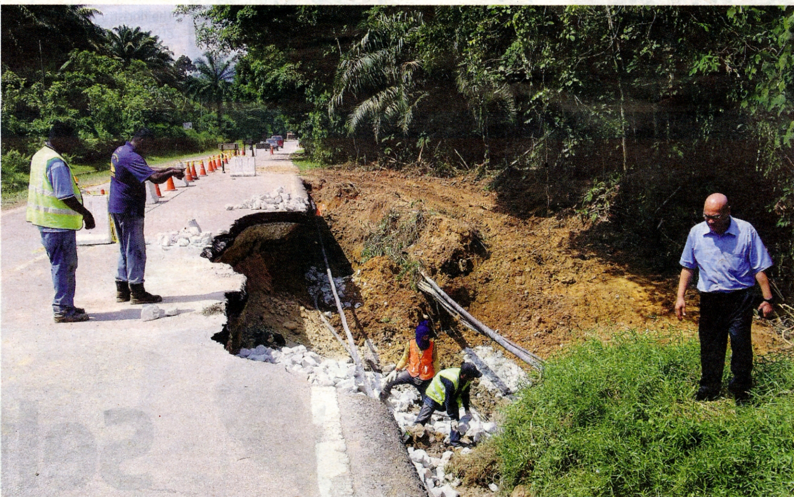
Dangerous: Contract workers working on the half-collapsed road in Jalan Sungai Kamin in Ulu Yam while Hisham (right) supervises.
