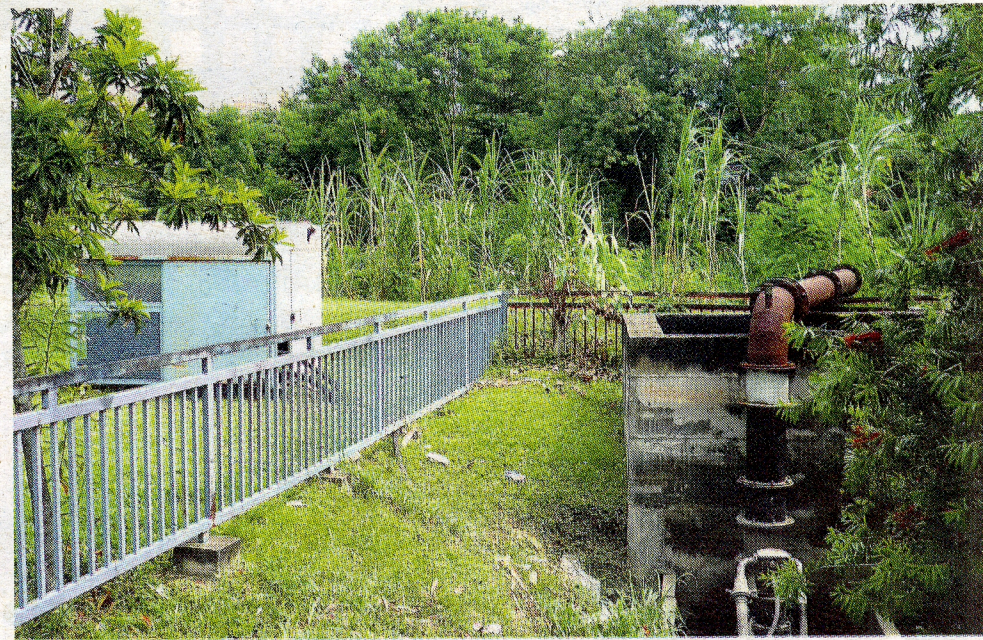
In need of repair: The pumps next to Sungai Kuyoh in Seri Kembangan malfunctioned recently leading to flood during the recent downpour.
