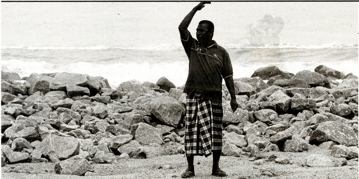
Sulaiman Muda standing near the collapsed section of the seawall in Kampung Tok Jembal, Kuala Terengganu, yesterday. Pic by Satiman Jamin
