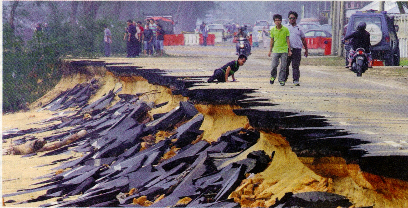
Ruptured link: Passers-by looking at a damaged road after it was hit by waves at Teluk Lipat beach in Dungun, Terengganu.
