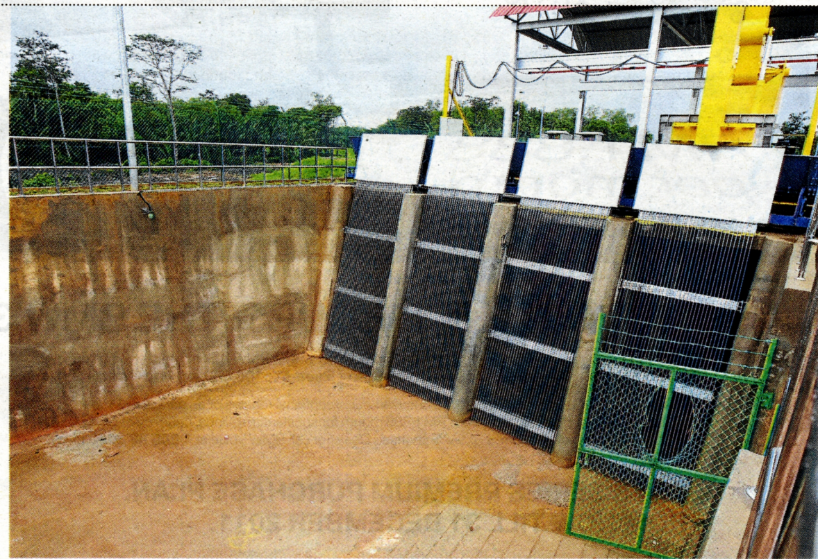
The water pumps at Tanah Putih to help alleviate the flood problem near Sungai Kuantan in Kuantan, Pahang. Pic by Azmaidi Abidin
