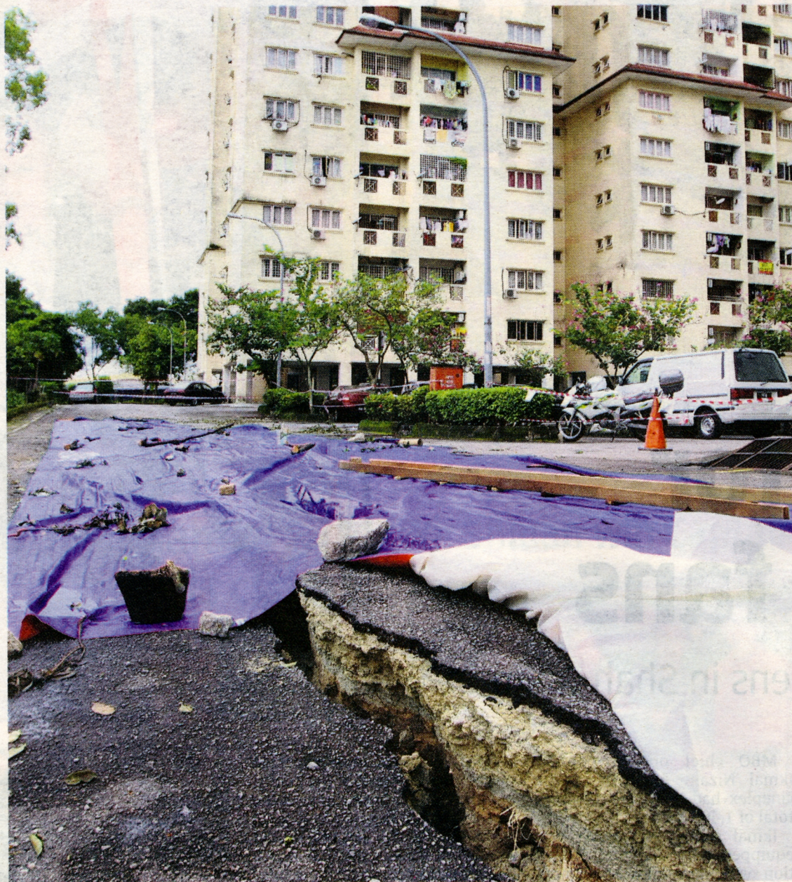
Serious damage: Residents are concerned over their safety.
