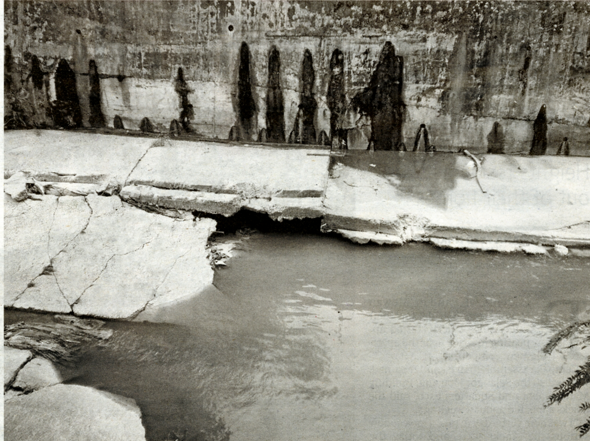
The damage to the retaining wall is believed to be the cause of the cracks.
