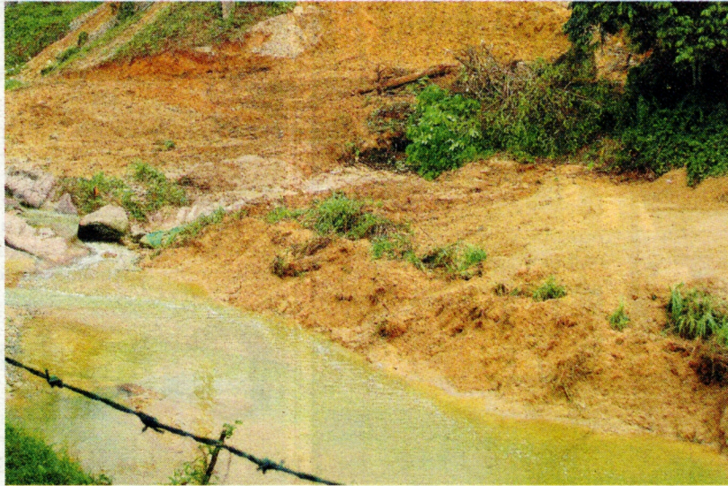
Work in progress: A filepic showing the riverbank where erosion took place was padded up with additional soil
