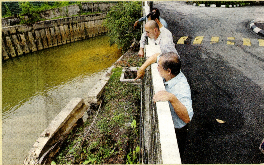
Segambut MP Lim Lip Eng (second from right) and residents inspecting the broken retaining wall along Sungai Penchala. —
