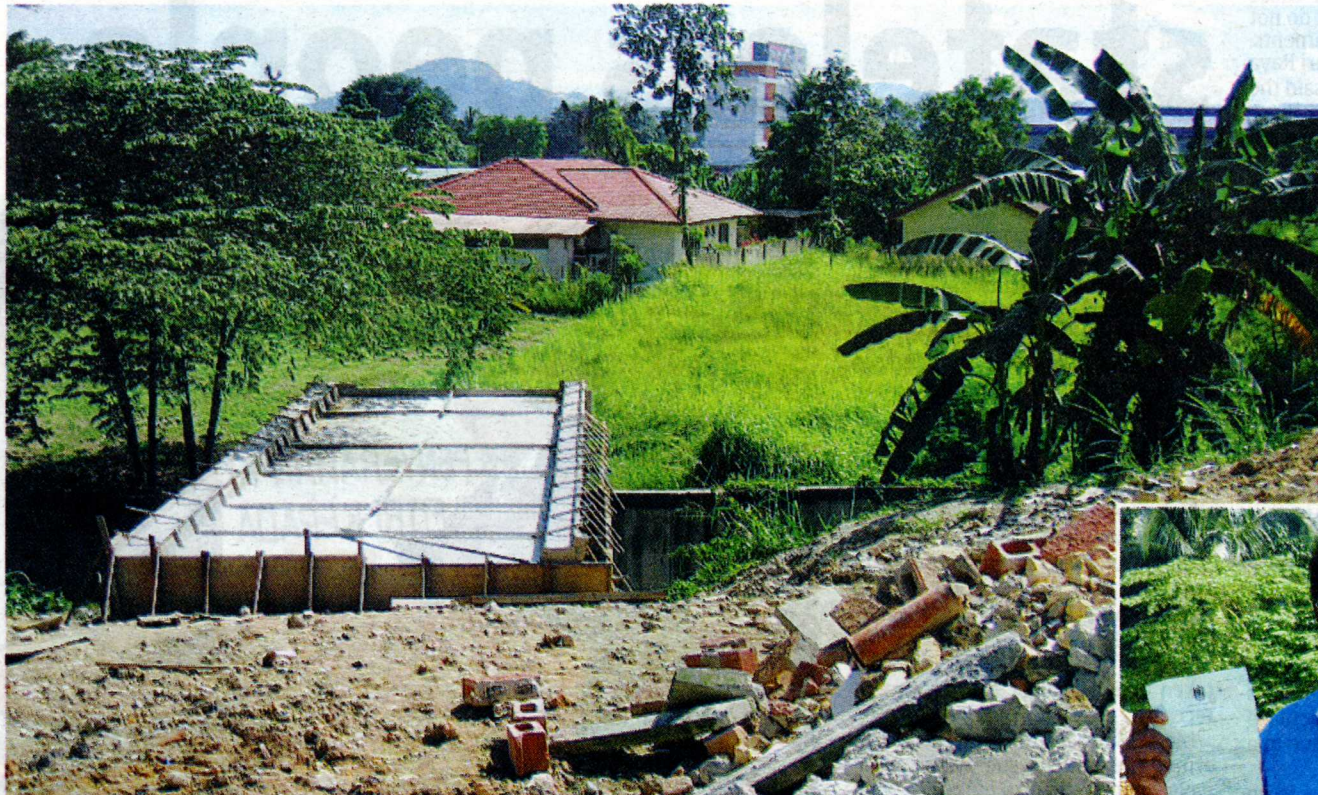
Left: The bridge built by a landowner across a monsoon drain to provide exclusive access to her house. Note the construction debris piled on the side of the drain reserve.
