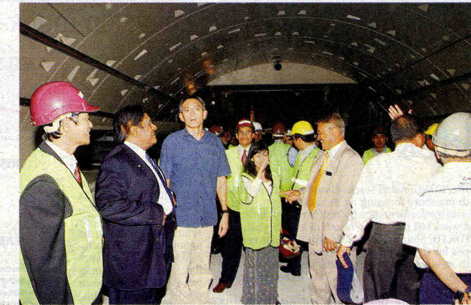
Samy Vellu (second from left) checking on the progress of work on the SMART tunnel yesterday
